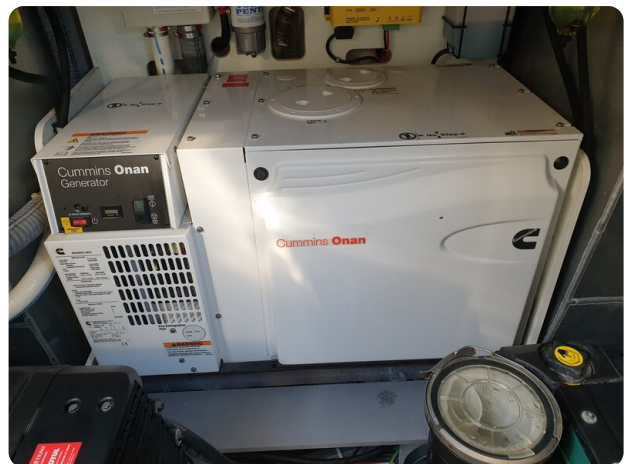
Beneteau MC5 generator
