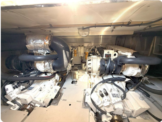
AZIMUT 55 Engine room
