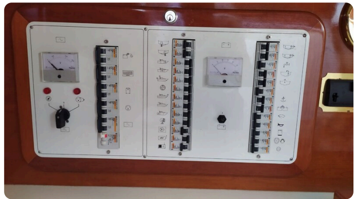
Apreamare 9 Open - Electrical Panel
